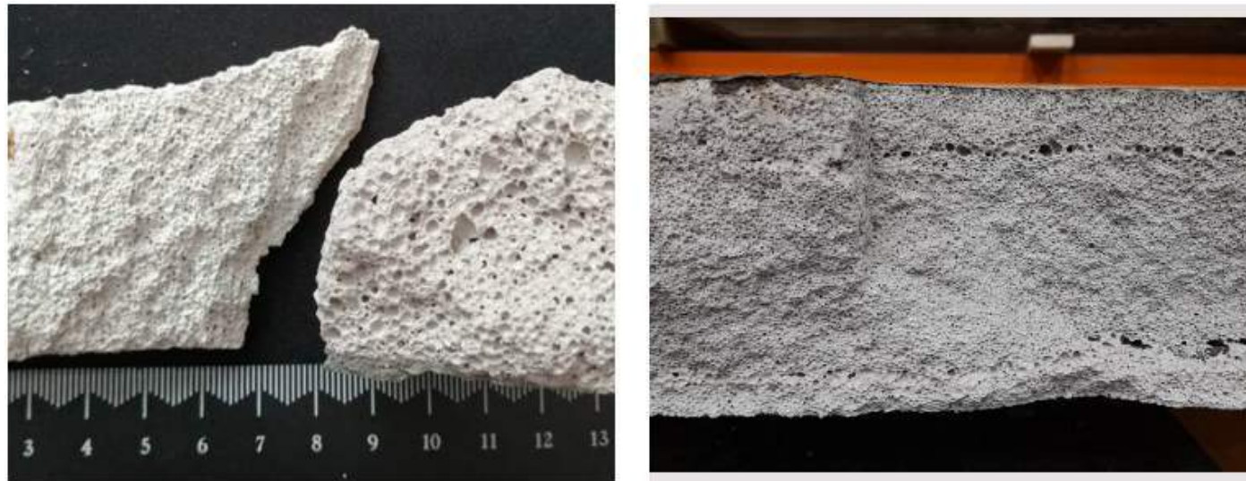
Figure 1 - Images showing physical properties of RAAC panels
